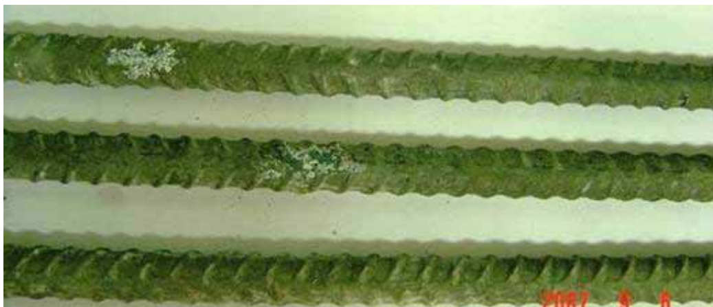
Figure 9 – Specimen B-Zn-45N-11 showing corrosion on top bar (top) and bottom bars (bottom)
