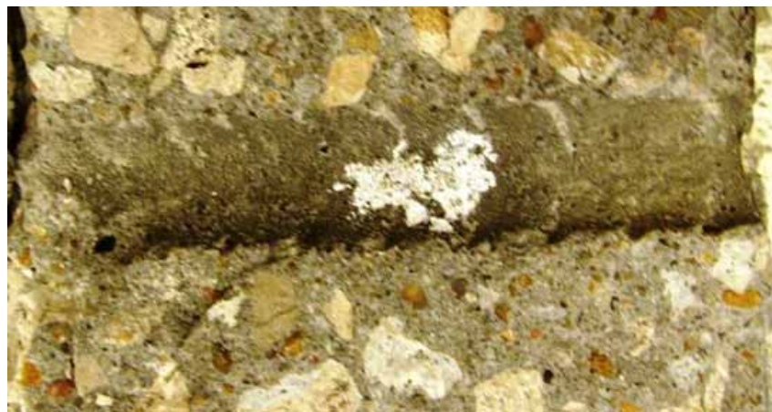
Figure 12 – Specimen B-Zn-45N-10 after autopsy. Visible staining appears on the concrete
